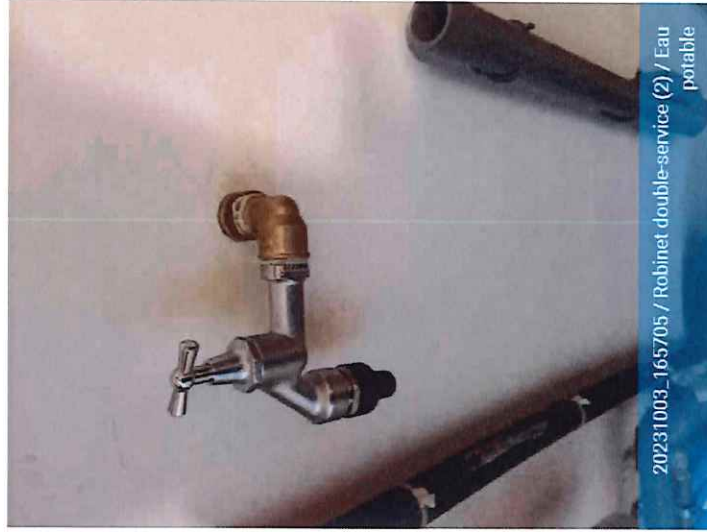
20231003_165215 / Robinet double-service (1) / Eau potable
